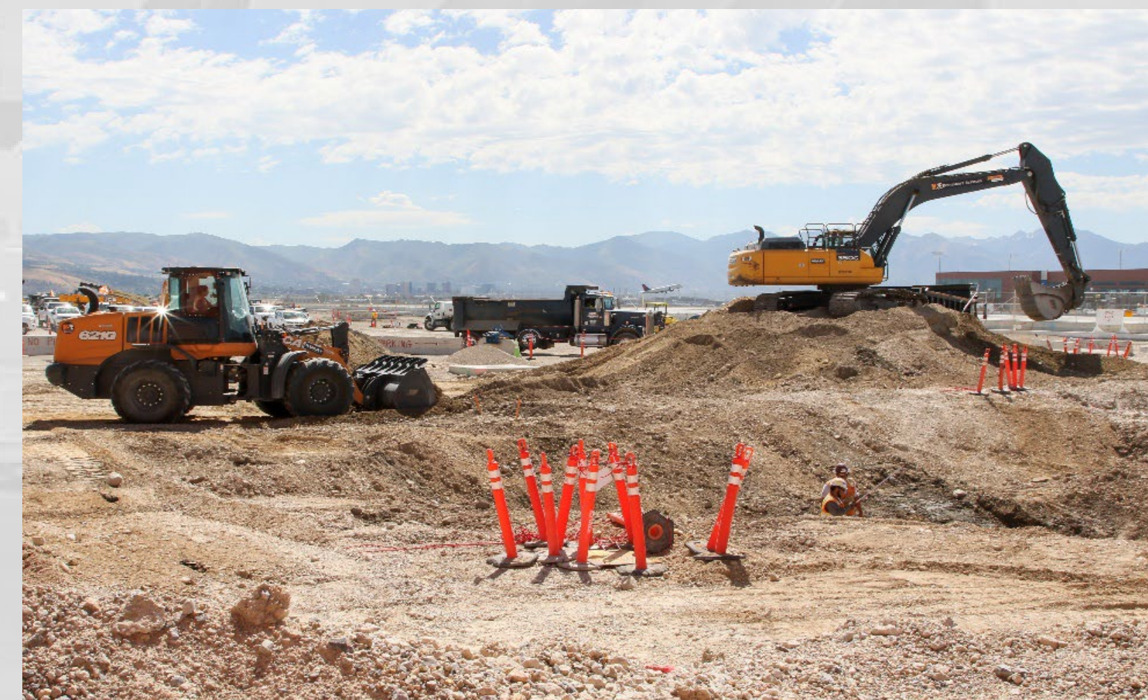
South Apron Hydrant Fuel Line
