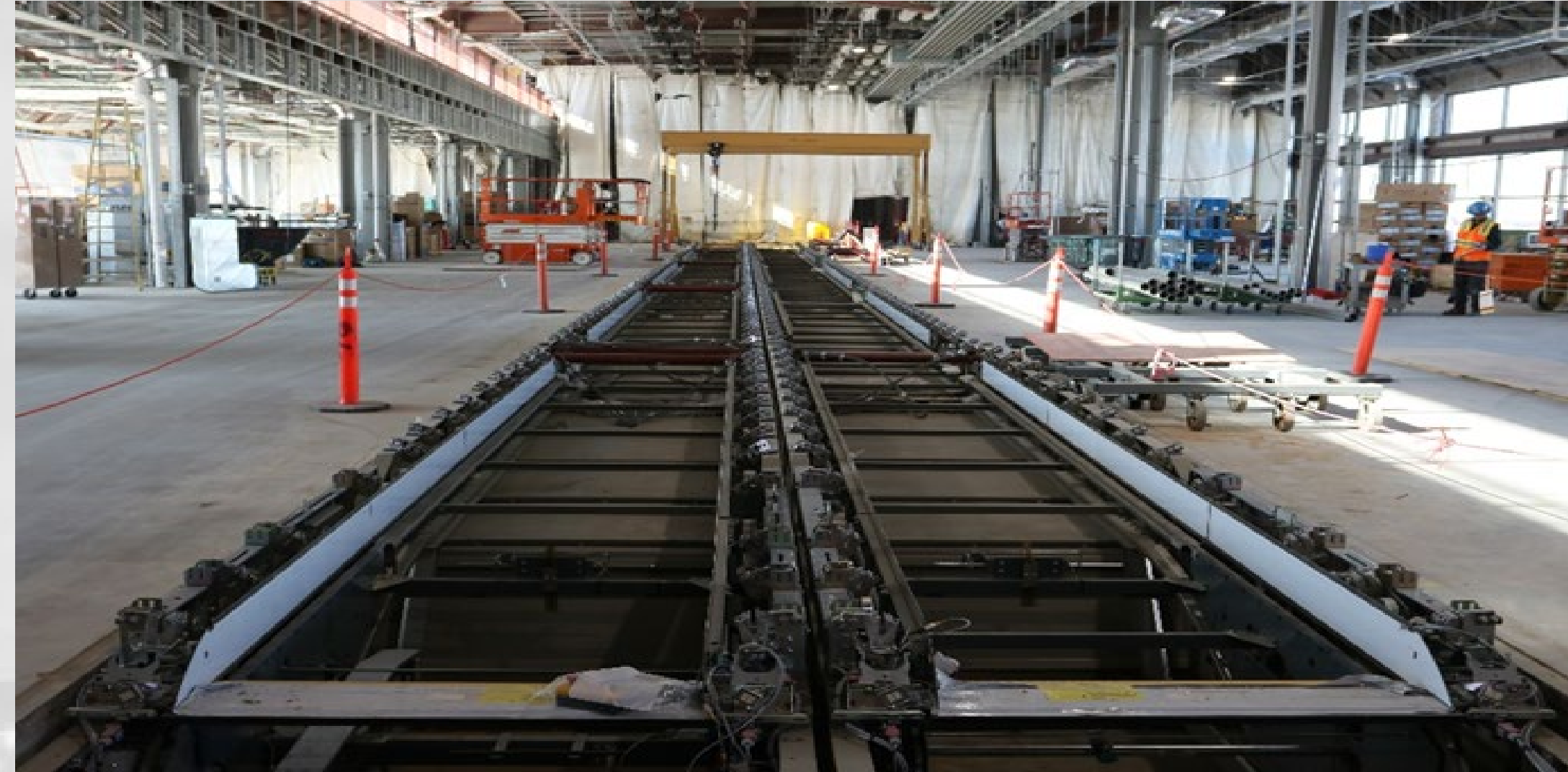
Level 2 Area C Moving Walkways
