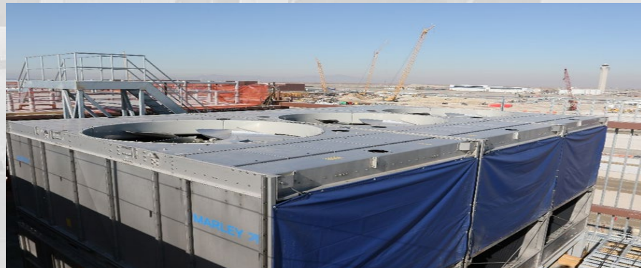
Area D Rooftop Cooling Towers
