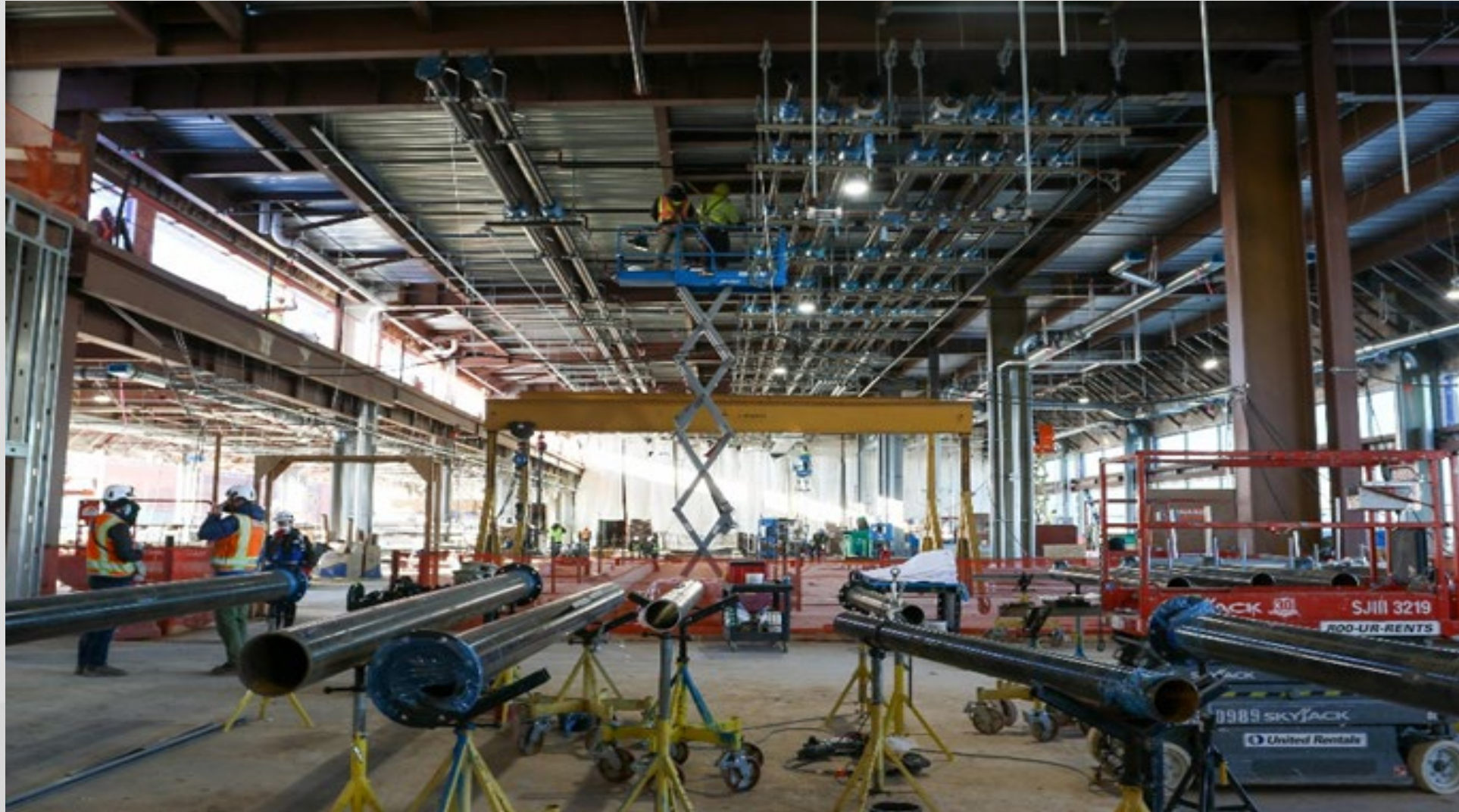
Level 2 Area B Hydronic Piping
