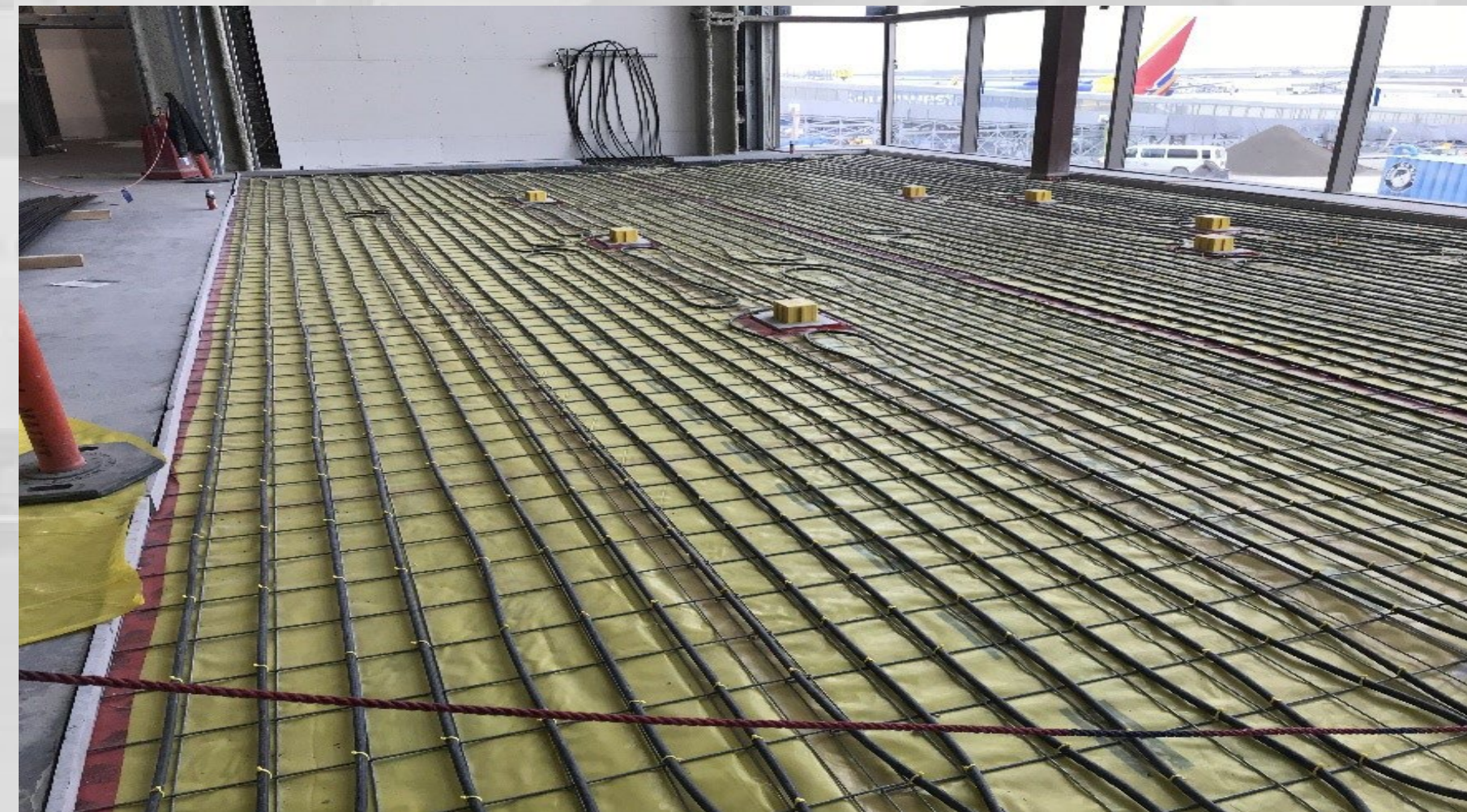
Area G Level 2 In-Slab Radiant Heating
