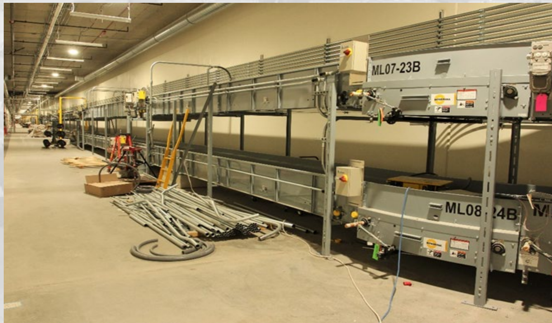
High Speed Baggage Conveyor
