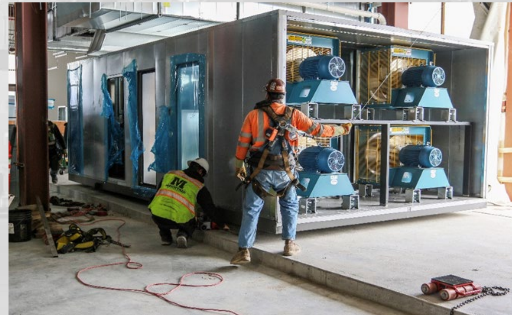
Level 3 Air Handling Unit
