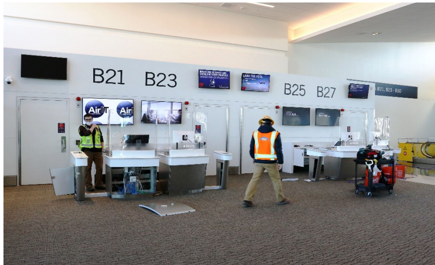
Bus Holdrooms IT Installation
