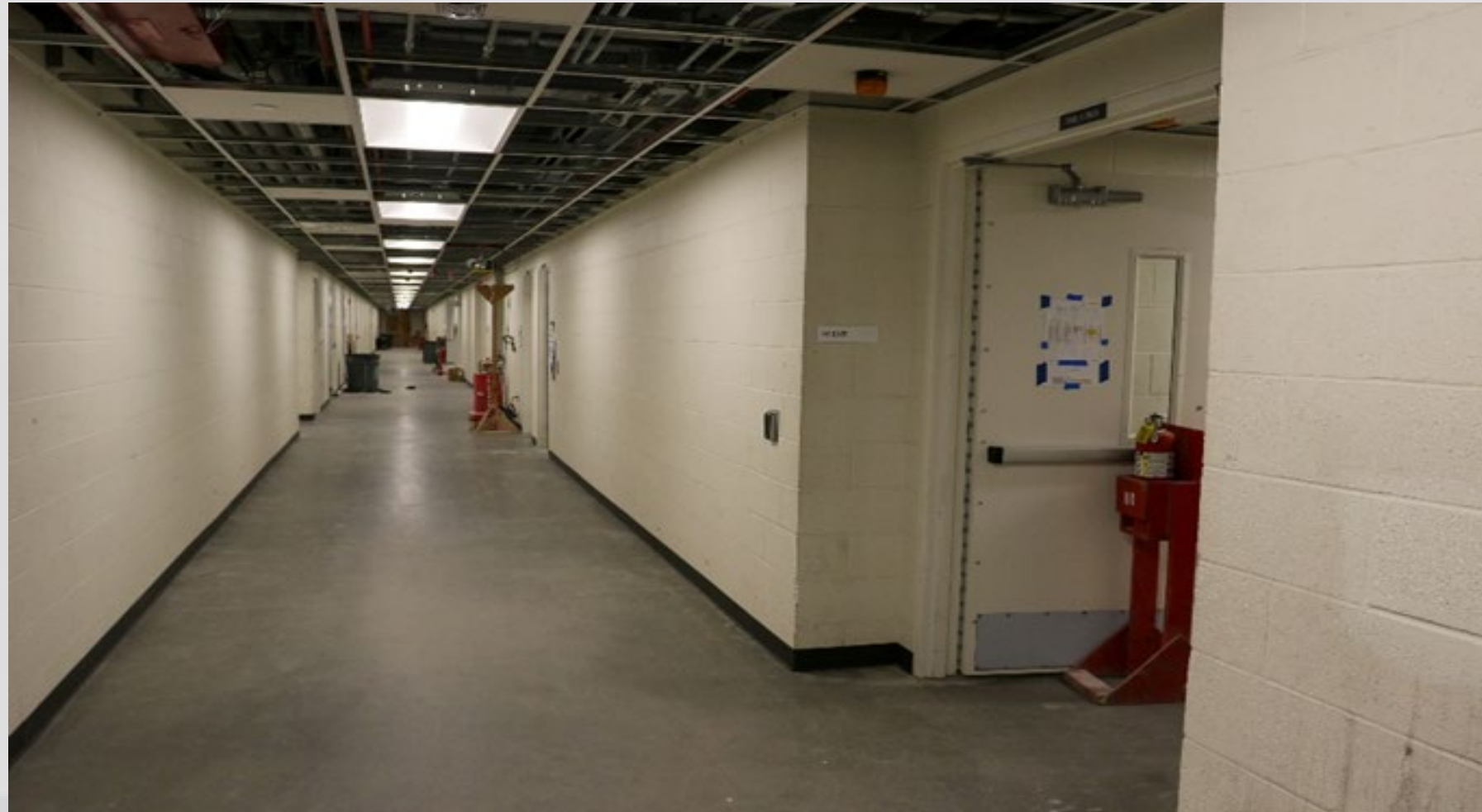
Service Corridor Ceiling Grid and Lighting
