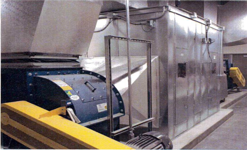
East Mechanical Room air handling unit in operation.
