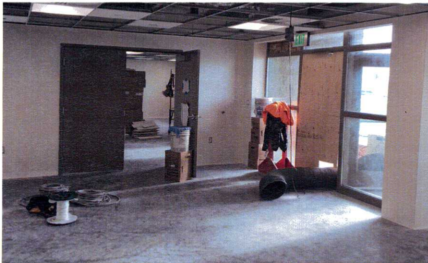
Interior Progress in RSS 'B' Admin Area. RSS B is the only building remaining requiring temporary heat.
