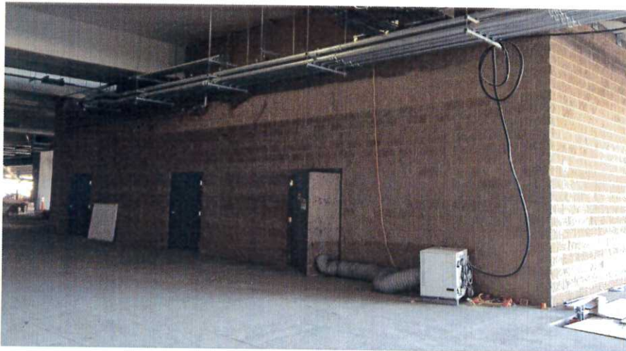
Parking Garage Electrical Rooms
