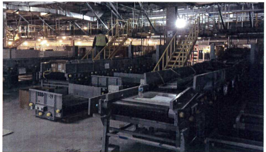
Baggage Handling System in Terminal CBIS
