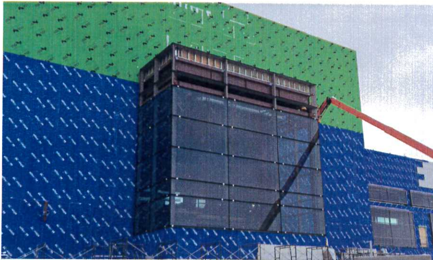
SCW Area 'E' Curtain Wall
