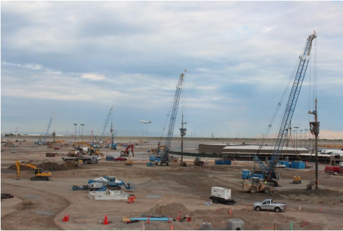
Cranes install stone columns to stabilize the ground and to meet seismic code.
