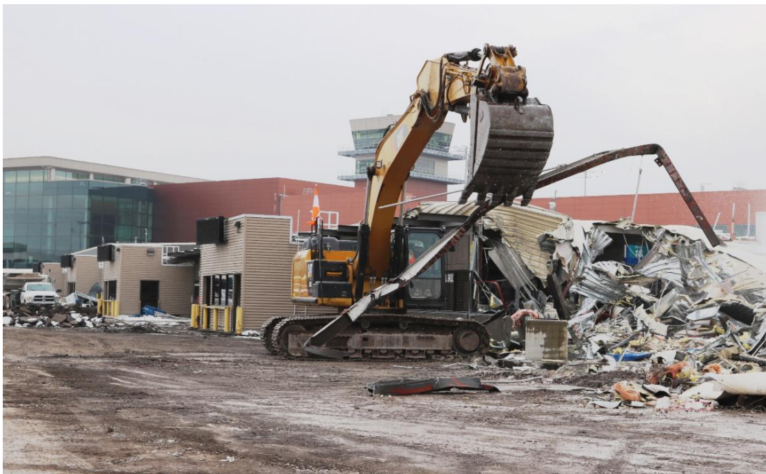
Concourse E was demolished earlier this year to makeway for The New SLC international gates.
