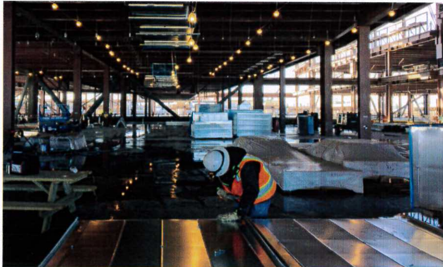
HVAC Ductwork in the Terminal
