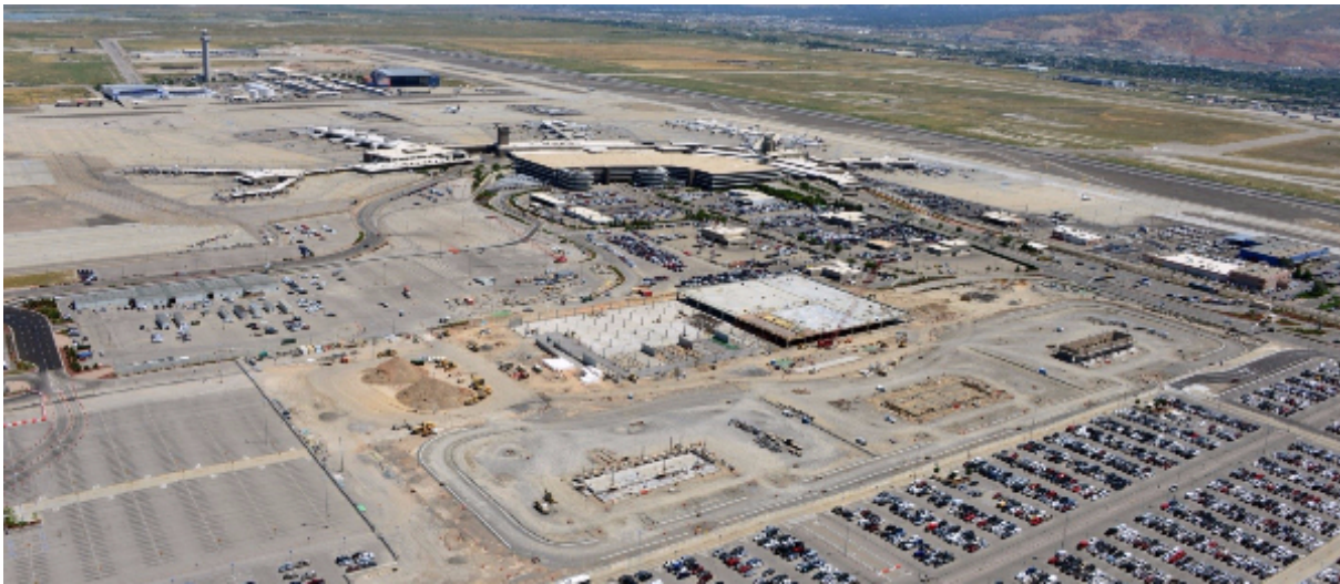
The first major project in The New SLC reconstruction program, visible in the center of the photo, is building Quick Turn-Around and Rental Service Site facilities for rental car agencies. Rental counters will remain next the new terminal, as they are today.
